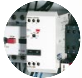
Protection ensures reliability of operation and safeguards your investment
